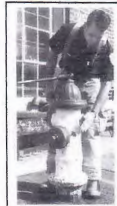
Example of testing a hydrant's draining ability. (Hall 387)
